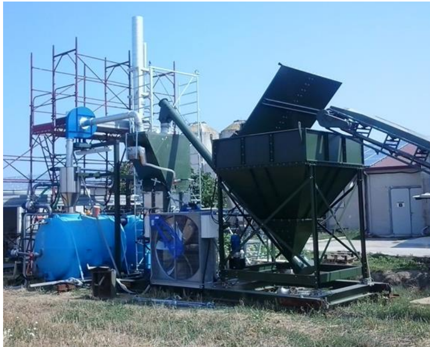
The CHIMERA prototype installed at F.lli Lorenzetti farm
